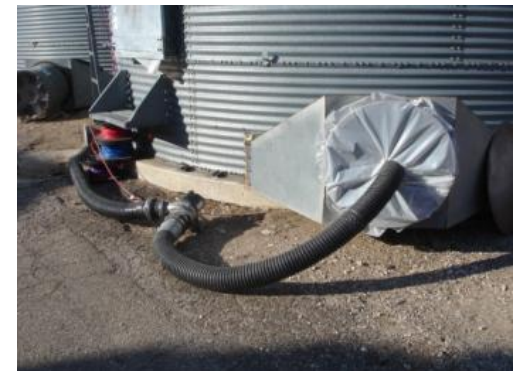
Sealed vent to bin aerating system
